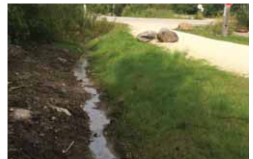
The Town of The Blue Mountains improved culverts at the Trail crossing near Grey Rd 40 to prevent wash outs. The Town also improved culverts near the round-about at Lora Bay and resurfaced the Trail at that location.
