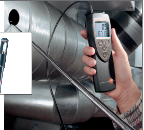
Monitoring air velocity in air conditioning ducts
