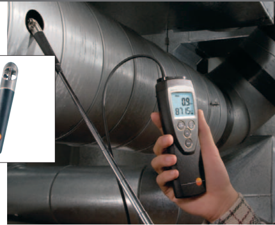
Monitoring air velocity in air conditioning ducts
