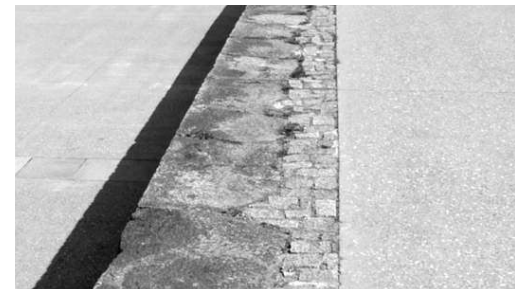
A photograph of the existing pier walls in Dún Laoghaire. The approach to restitching historic fabric to a new contemporary surface material that is cohesive, yet distinct.
