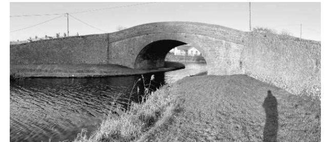
The Whitehall (Bury) Bridge where the Grand Canal meets the Canal Spur
