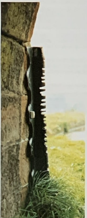
Grooves cut by tow ropes in a typical cast iron bridgeguard
