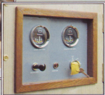
The simple control panel and switches.
