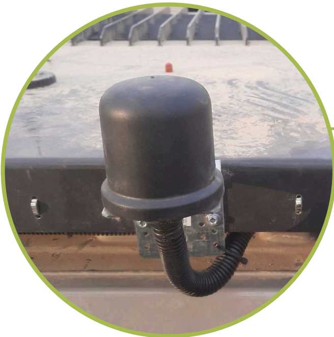
External LTE antenna
