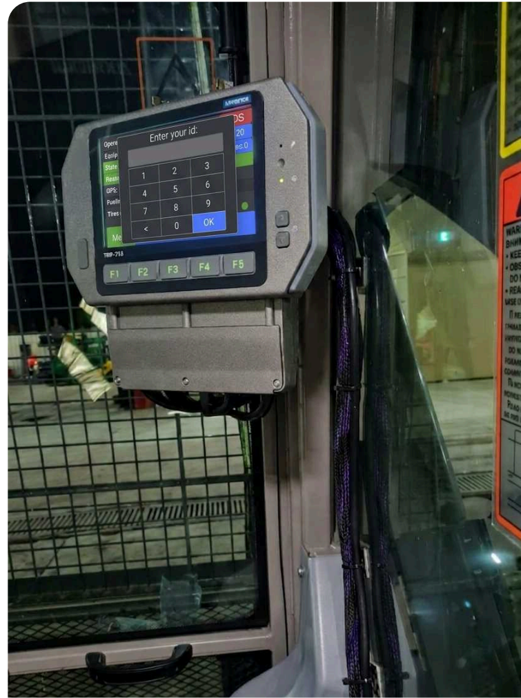
Computer installed in the cabin
