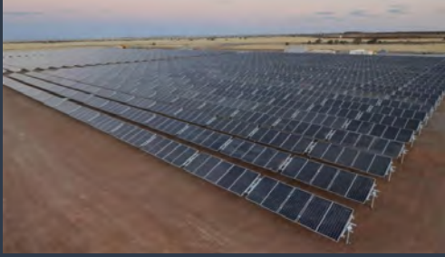
3MW Cannington Mine Solar Farm, McKinlay QLD
