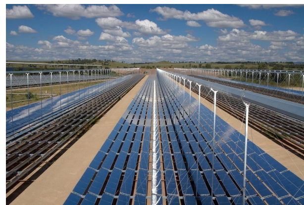
9 MW solar thermal farm, Liddell NSW
