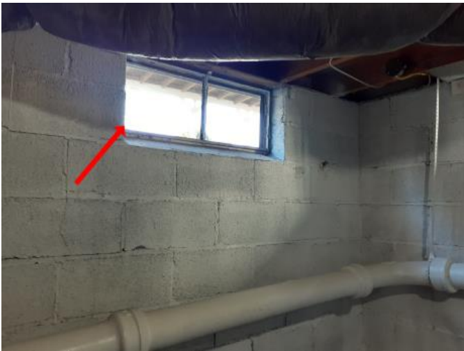
Missing glass panes
