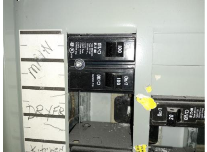
Main shut off
