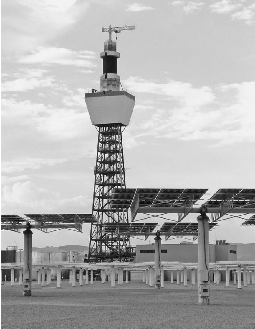
FIGURE 32.1 A solar tower power plant in Daggett, California.
