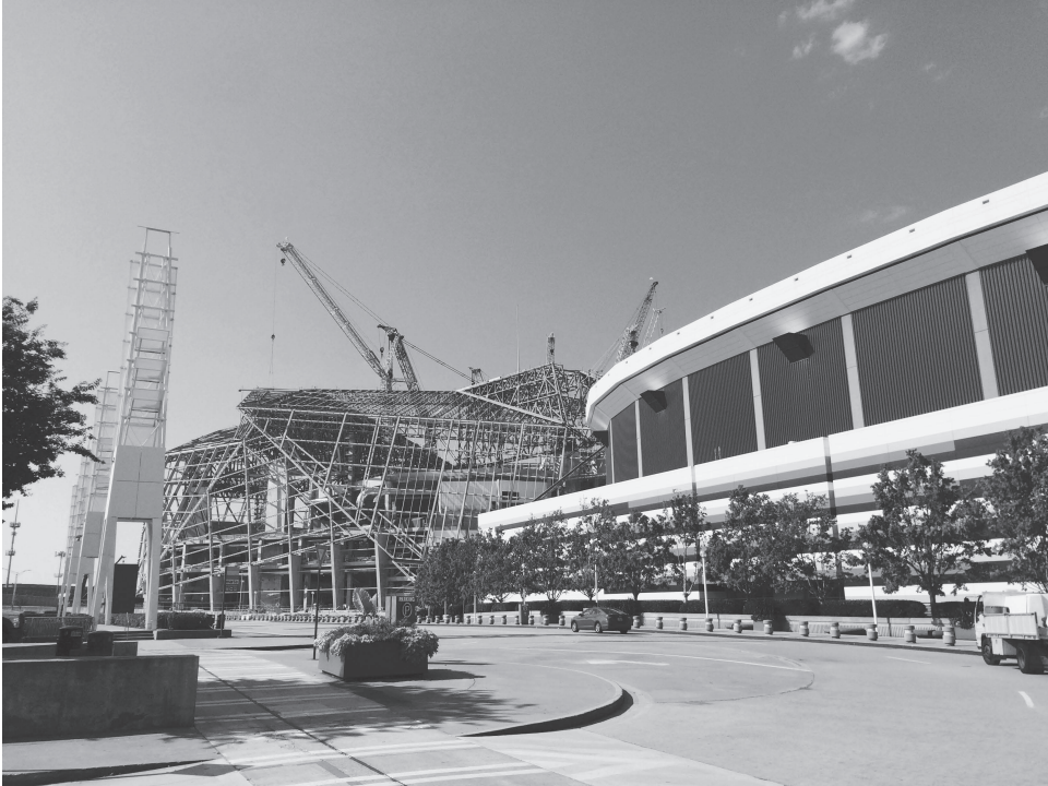
Figure 34.1 Mercedes-Benz Stadium in Atlanta, Georgia, pictured under construction in 2016. The new home to the Atlanta Falcons NFL team replaced the Georgia Dome, pictured in the foreground
