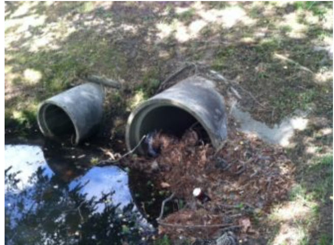
Accumulated debris at this outlet could impede flow leaving the pond, impacting its ability to manage large rain events. Once noted, the pond owner should clear as soon as possible to avoid clogging. C. Guinn Wallover, ©2020, Clemson Extension
