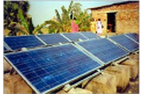
Fig.30. Rooftop PV modules in West Bengal, India used to power lights and refrigerators that contain vaccines and medicines. Source: US Dept of Energy
