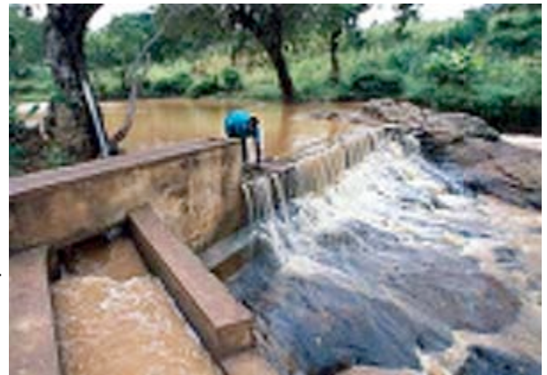
Figure 36. The Tungu-Kabri micro-hydro power project in Kenya run by Practical Action East Africa. Source: Practicalaction.org
