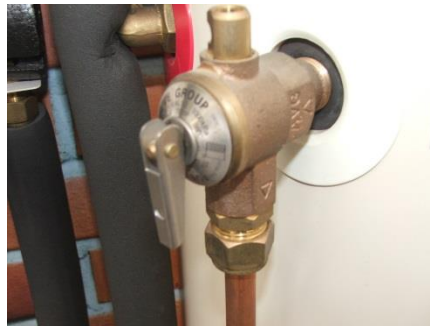
Temperature and pressure relief (T&PR) valve © NMTAFE 2014
