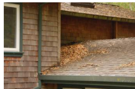
Replacing siding "locally," in areas where it meets the roof on a complex roof design, such as that shown here, would be more affordable than "global" replacement. Source: Stephen L. Quarles
