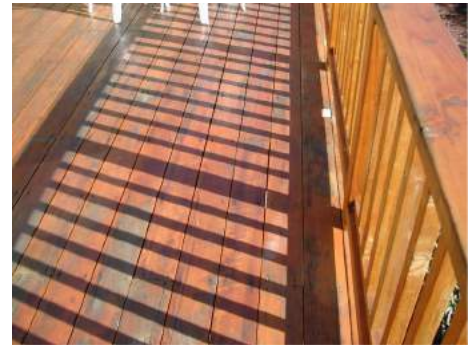
A deck with wood (combustible) deck boards. Source: Stephen L. Quarles
