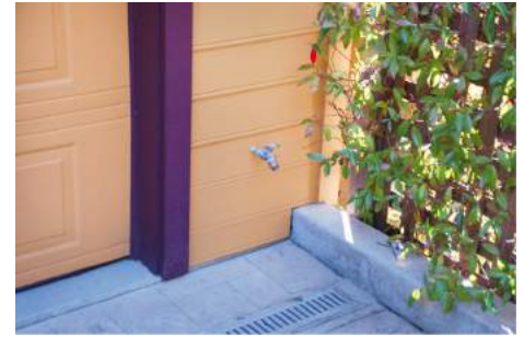
A noncombustible lower course of siding was used in this installation with otherwise combustible siding used in the higher courses. Source: Stephen L. Quarles
