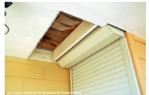
A horizontal enclosure, such as that shown here, can result in moisture-related degradation of wood and metal fasteners when deck boards are used.
