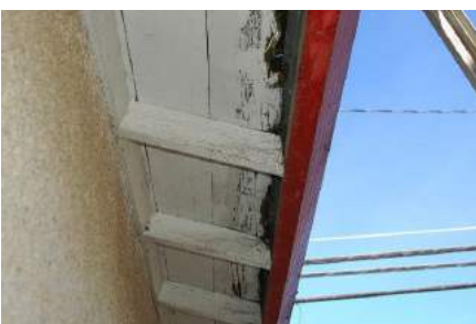
Decayed wood at the roof edge—more readily ignited from any flaming exposure resulting from burning debris in the gutter. Source: Stephen L. Quarles
