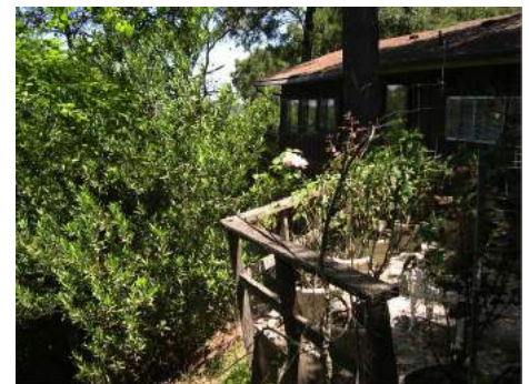
The defensible space on this property could be improved by removing vegetation to minimize the opportunity for fire to burn directly to the home. Source: Stephen L. Quarles
