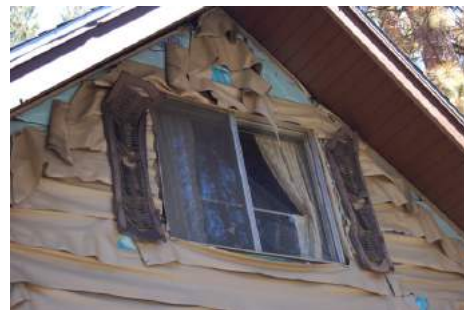
Deformed vinyl siding from a radiant heat exposure from a nearby burning home. Source: Stephen L. Quarles
