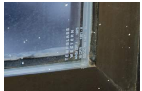
Etched “bug” in the corner of a window indicates that the window glass is tempered. Source: Stephen L. Quarles
