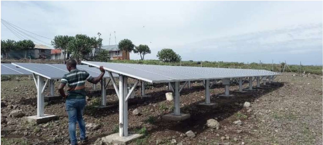
Photo 5: mini grid at Ringiti Island. Photo credit: Rosebella Nyumba
