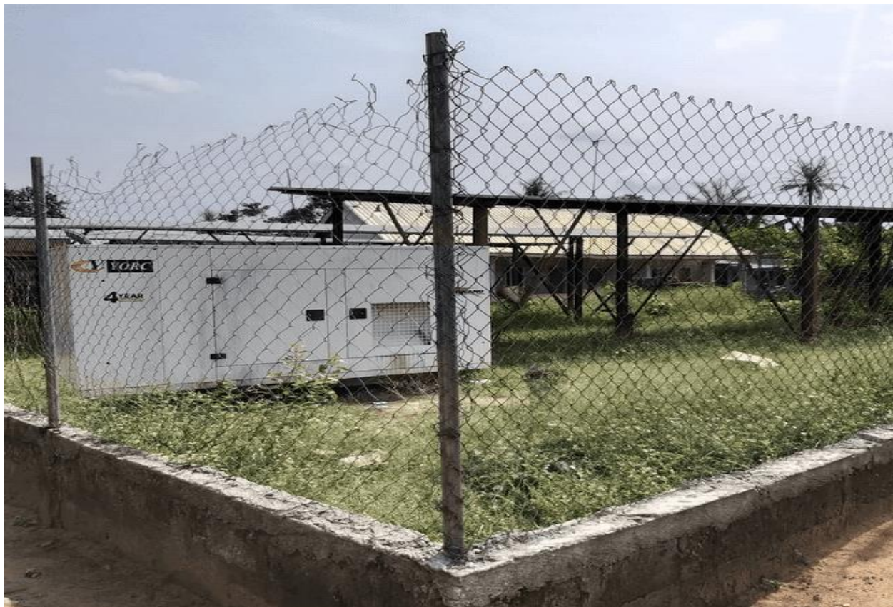
Figure 7: Ozuzu community mini grid plant
