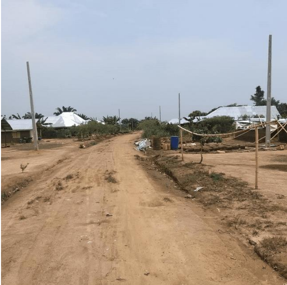
Figure 6: Poles waiting to be energised
