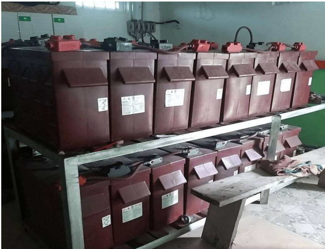
Figure 10: Akpabom mini grid battery bank
