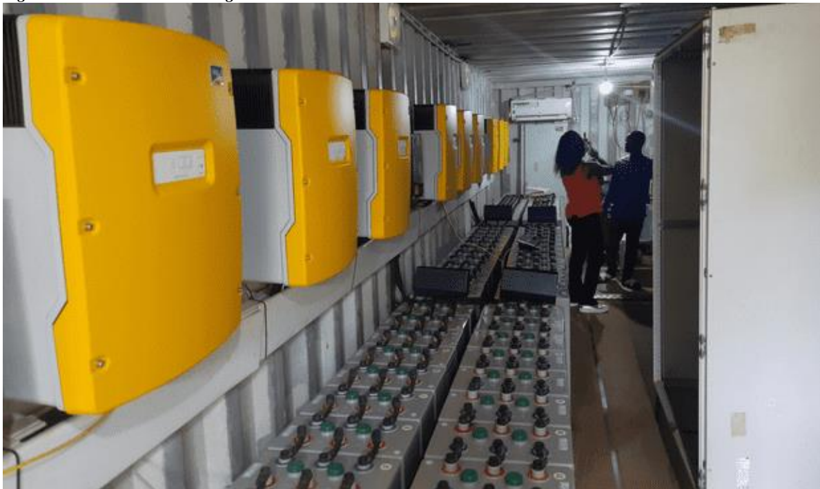
Figure 19: Gbamu Gbamu mini-grid battery bank
