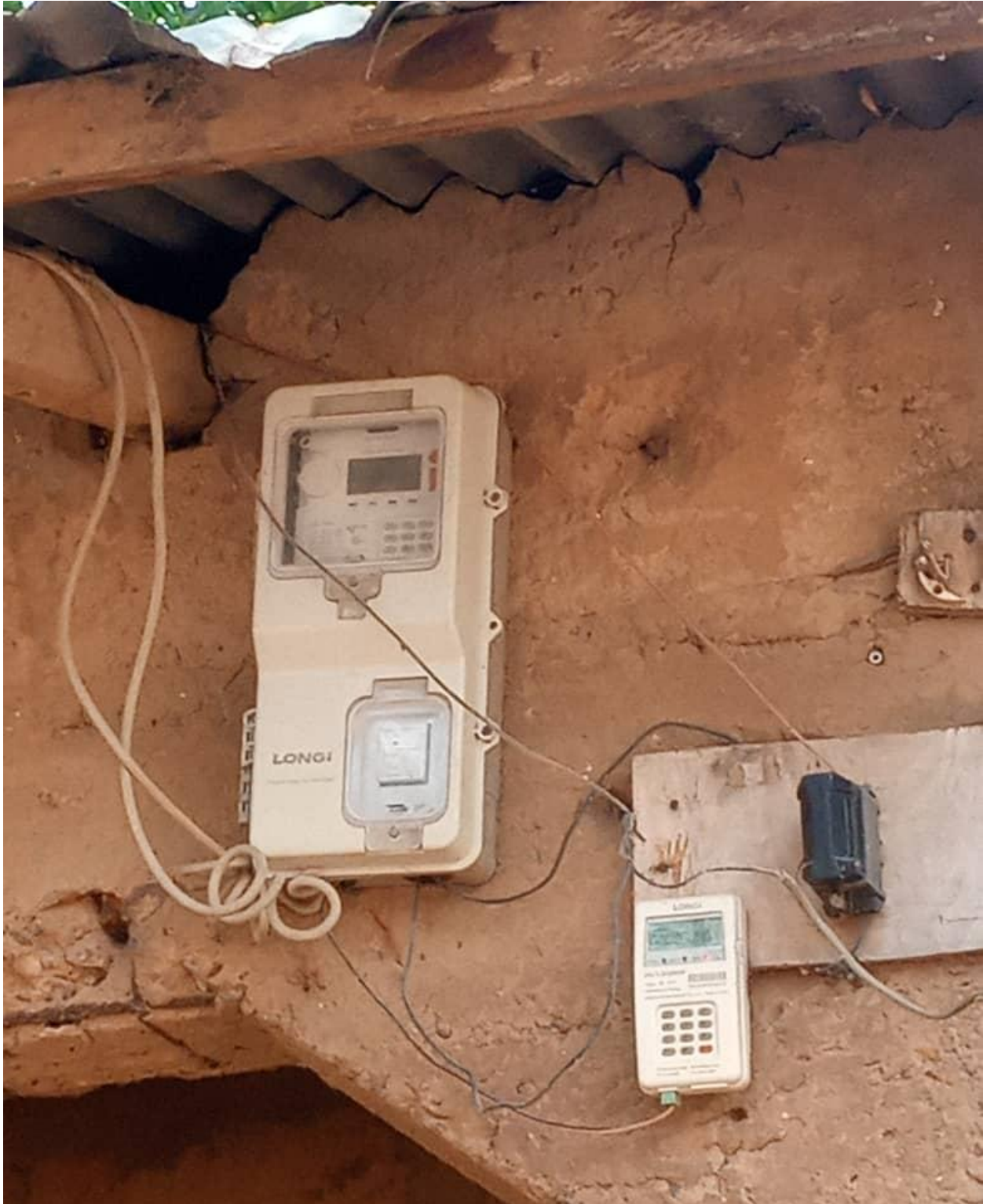
Figure 15: Sample electricity meter at Dakiti community
