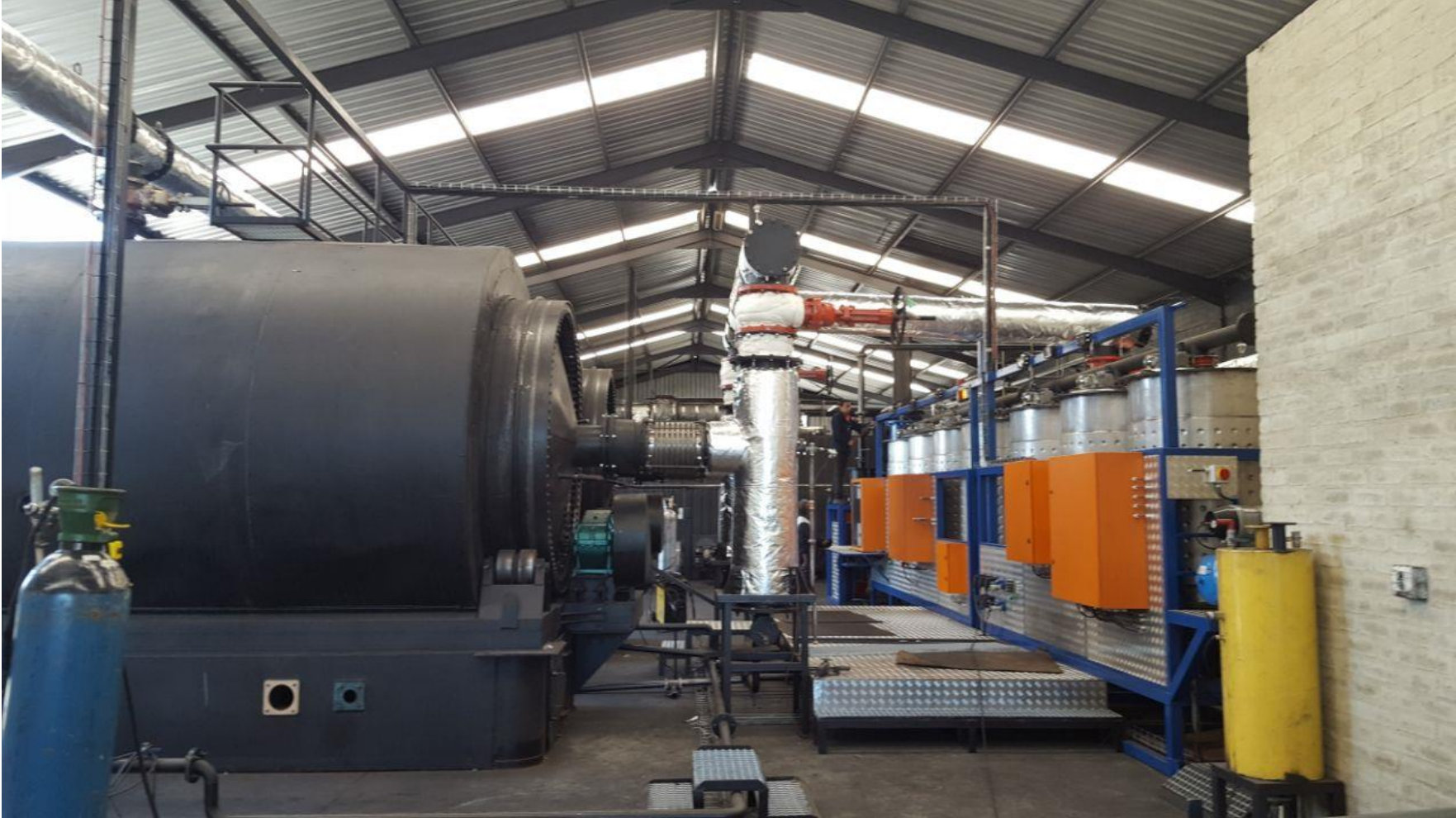
EXISTING PRIVATE-OWNED PLANT AT BOT RIVER, SOUTH AFRICA
