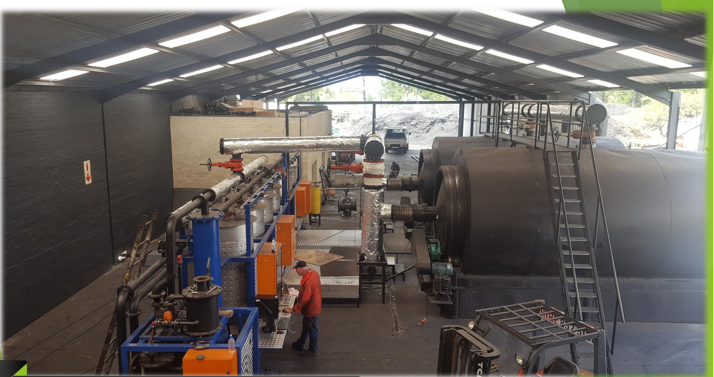
Commissioning of Botrivier Plant 15
