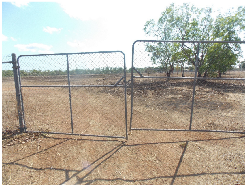
Gates to the oval in sad condition waiting for funds to repair them and the oval grounds behind them.
