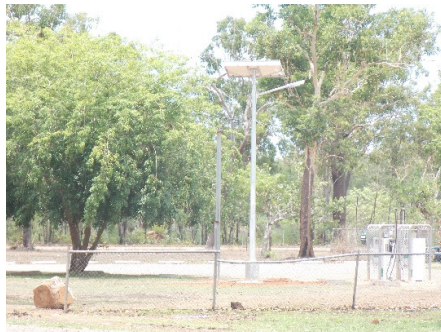
Solar street light installed by Belyuen Council Civil Works staff
