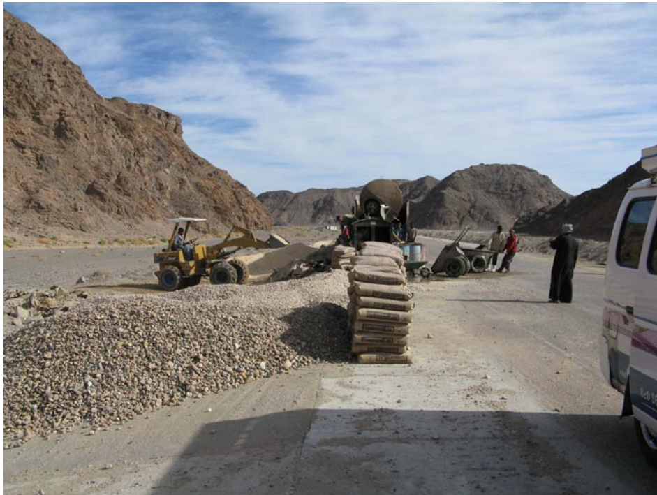
Fig. 22. Reinforcing the main Quft – Quseir road in the Wadi Hammamat against flash-floods (15 November 2011)
