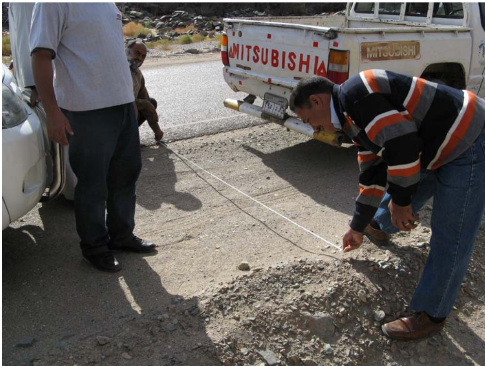
Fig. 23. Works manager measuring the extent (2.75 m) of horizontal road reinforcing in the area of key archaeology
