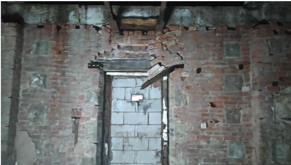
Photograph 12: Lodge 1 - Failed Timber Lintel / Unstable brickwork
