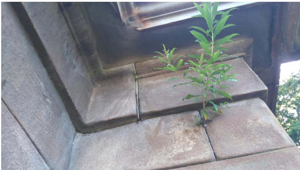
Photograph 10: Missing pointing / vegetation growth
