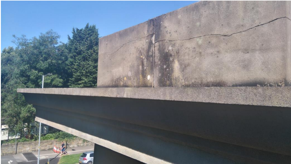
Photograph 7: Horizontal cracking to coping stones in arch at high level
