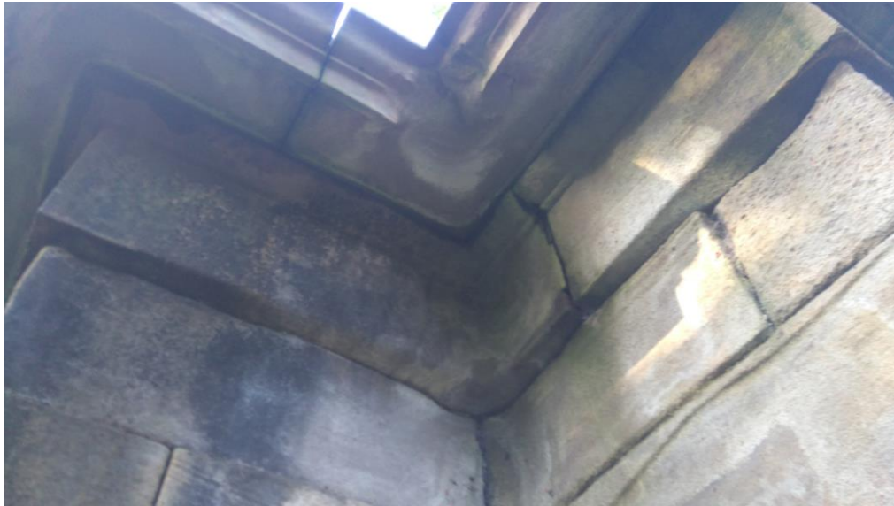
Photograph 9: Erosion Of Stonework / missing pointing
