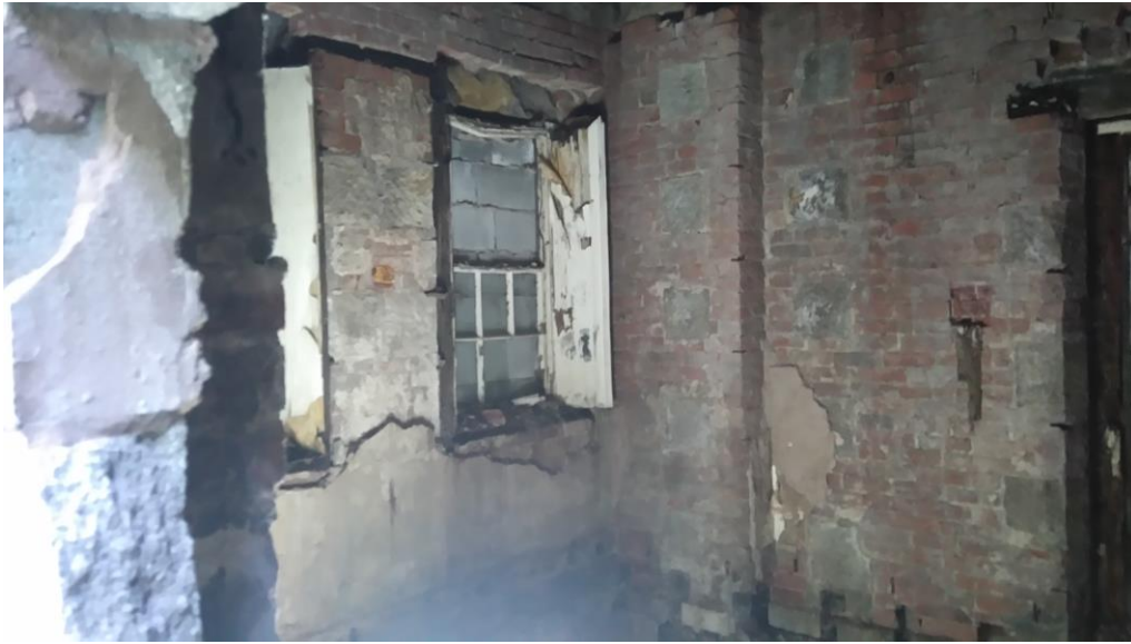
Photograph 13: Lodge 1 - Wet Rot To Timber Window Frames
