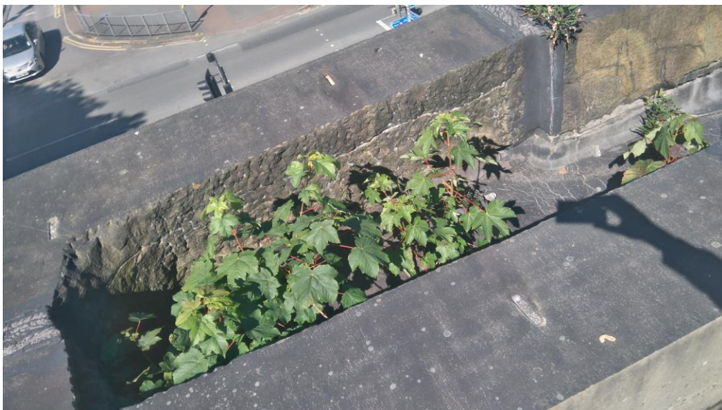
Photograph 8: Saplings / Vegetation growth on asphalt archway roof
