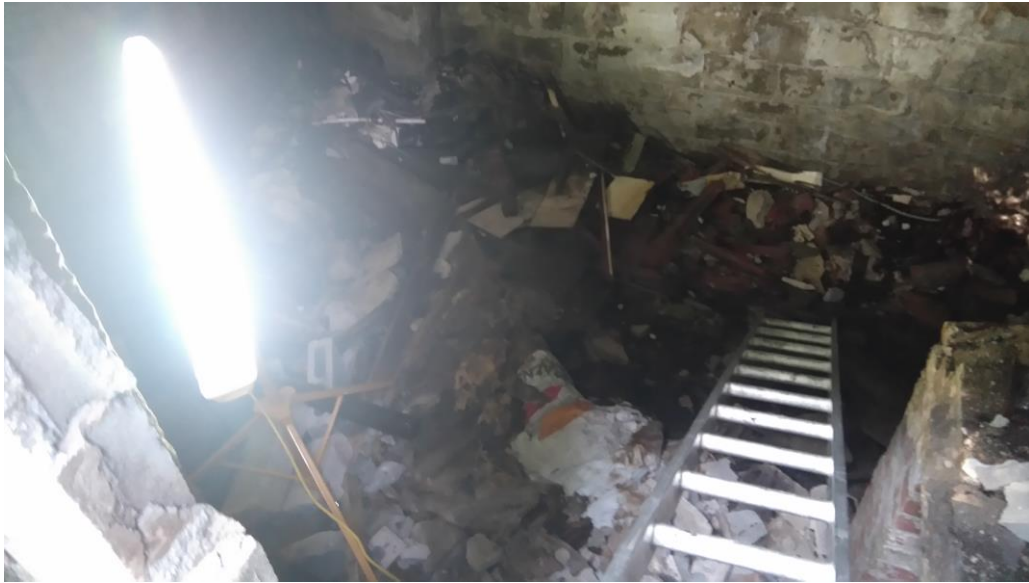
Photograph 15: Lodge 1 - Timber Joists / Debris in Basement Area
