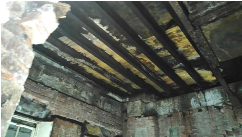
Photograph 14: Lodge 1 - Mould to underside of roof structure / Cast iron beam upon unstable brickwork
