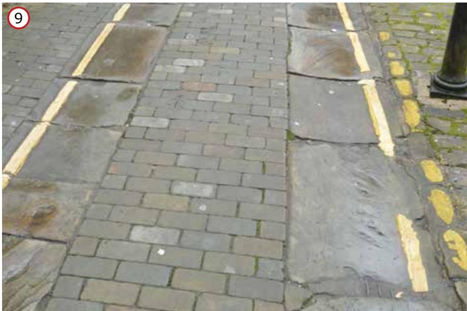
Sandstone setts and slabs are a common finish within Rowbottom Square, Bretherton Row and Arcade Street.
