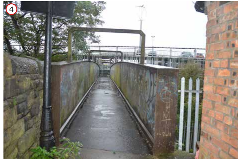
The existing footbridge is covered in graffiti and aesthetically is unwelcoming. This forms an under utilised route to Wigan North Western Train station.
