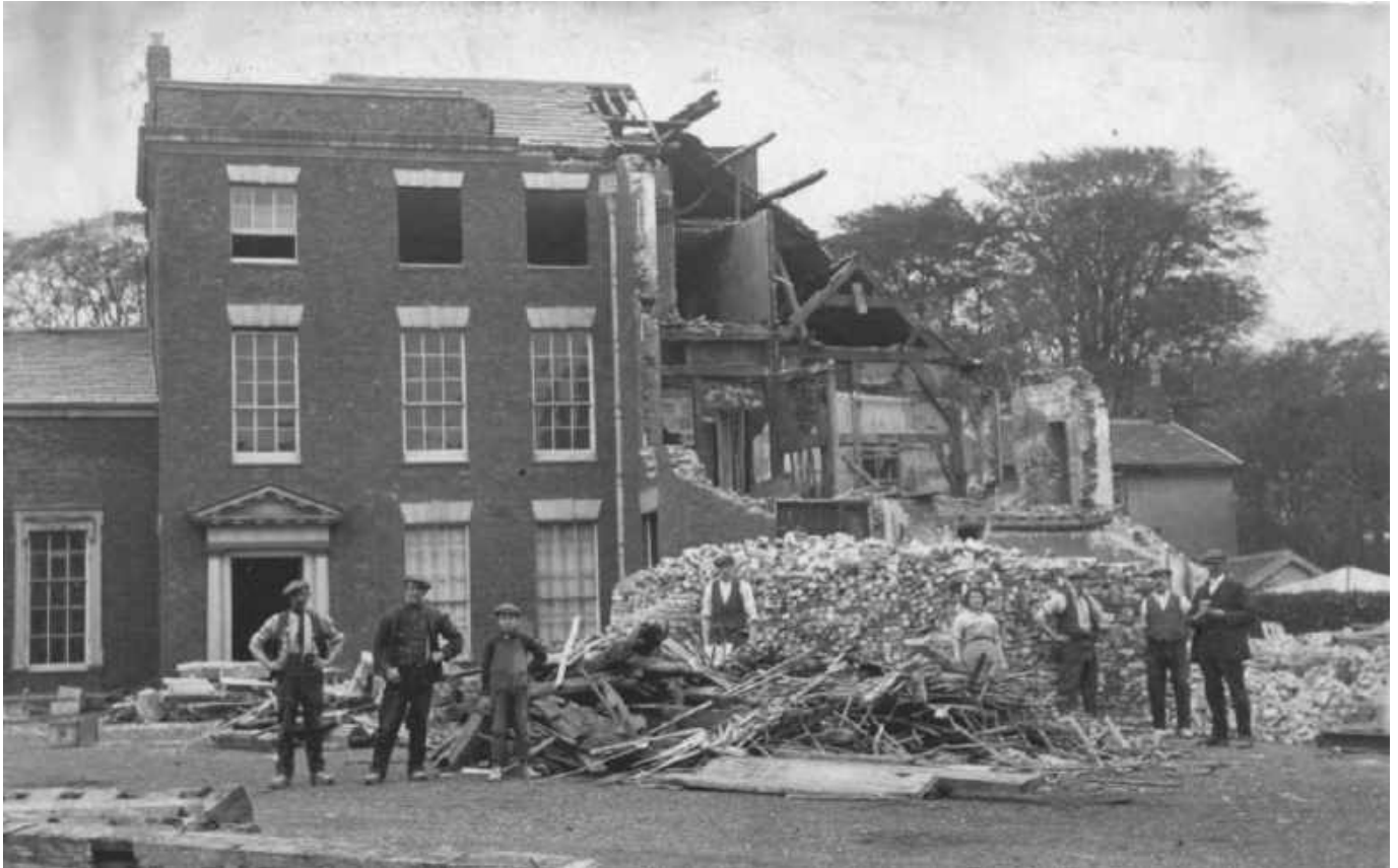
The Tudor Hall and Chapel being demolished in 1923. The valuable wood panelled rooms had been removed
