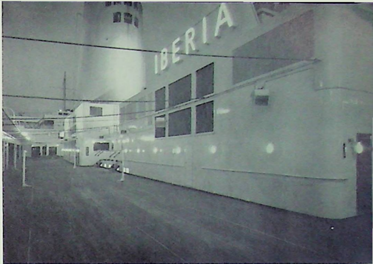
Lacent lighting fittings made by Heyes & Co. Ltd. installed on the "Iberia"
