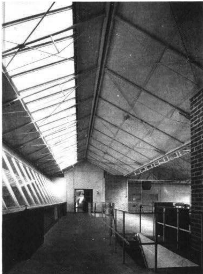
View showing roof over stores, giving access to workshops; this space is also used as an exhibition area.
