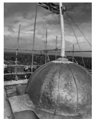
Completed restoration work on the copper dome at the top of the cupola on Leigh Town Hall
