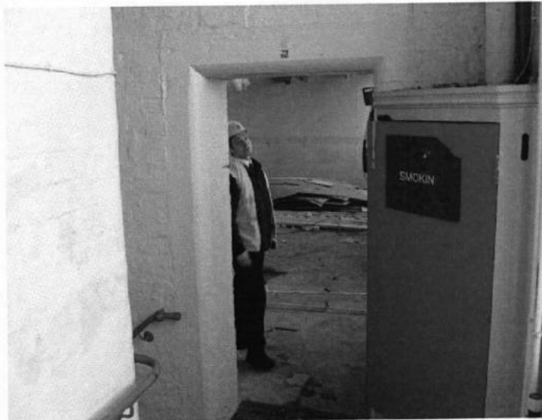
Fig.25: historic dry riser in corner of south-east stair tower (block B)
