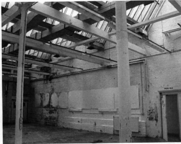
Fig.24: phase 2 weaving shed interior, looking north-east (roof structure proposed for demolition, wall to be retained and cleaned)
