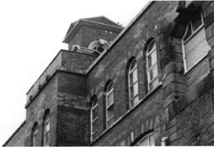
Fig.19: view of stair tower cupola and water tank, with taking-in door on north-east elevation (block B)
