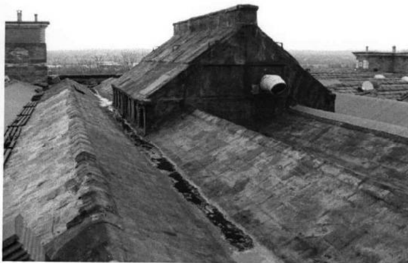
Fig. 27: glazed roof- lantern over former engine house, viewed to south- west (block B)
