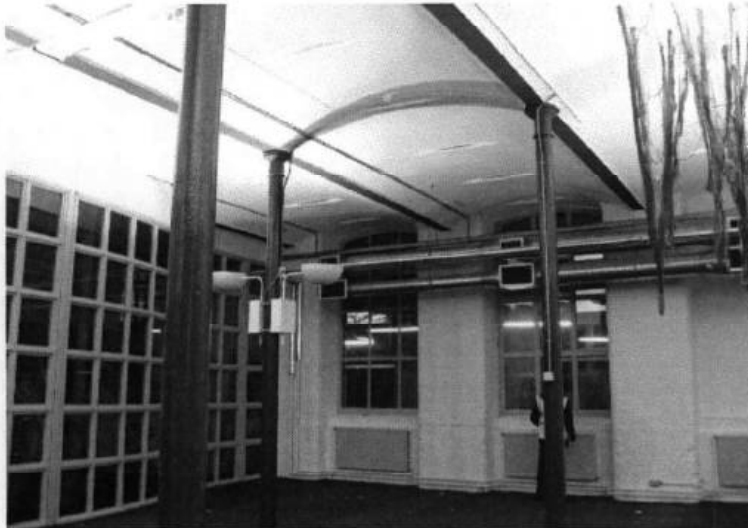
Fig.20: typical ground floor mill interior (block B), with brick vaulting and one new and one original (to left) window
