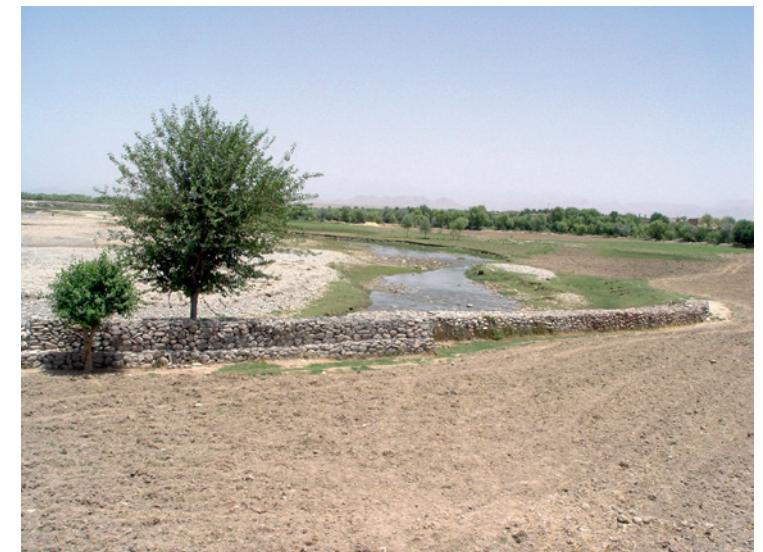
A road constructed in Uruzgan, Afghanistan, that at the same time strengthened an irrigation inlet
