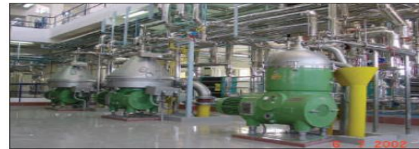
(i) A piping network in an industrial facility.
