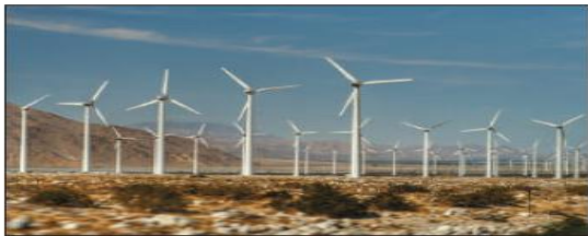
(g) Wind turbines
