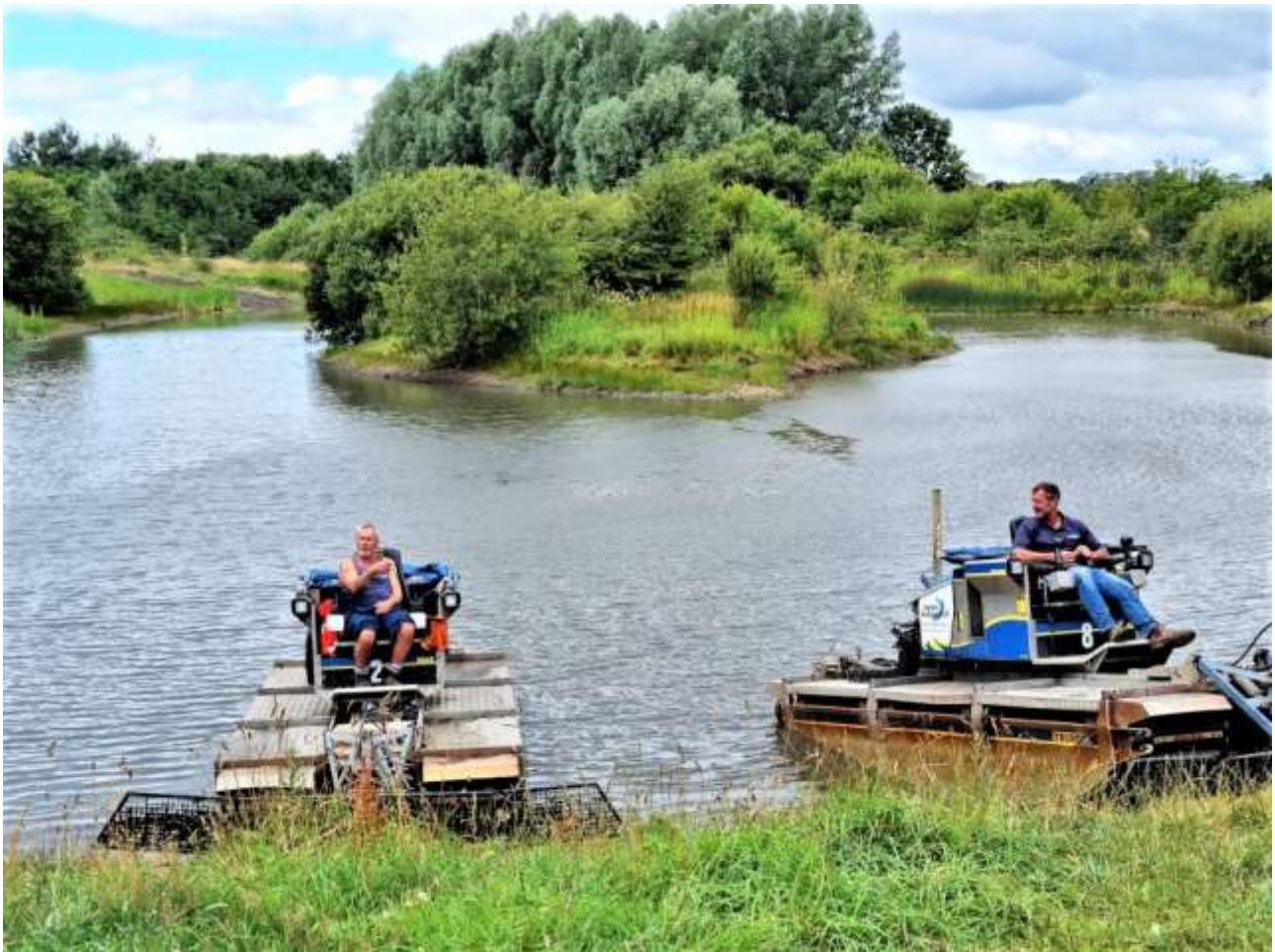
July 29 2021: Job Completed in 4 days: the pond is now looking like a pond again
