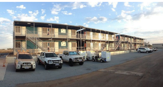
Project Village Accommodation Upgrade Client Grounded Constructions Scope FMG Hamilton Village Refurbishment Value $600K
