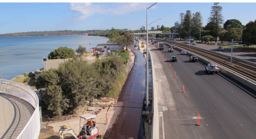
Project Main Roads WA - Kwinana freeway widening Client Smartways Alliance Scope Street Lighting, Civils and ITS Value $900K
