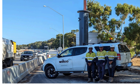
Project Mitchell Freeway Smart Freeways Client Intelligent Freeway Alliance Scope Street lighting, Intelligent Transport Systems Value $1.4M
