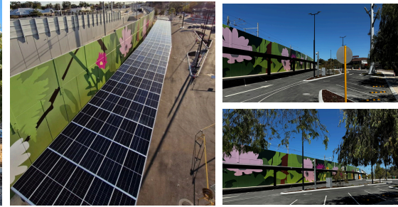
Project Bayswater Solar Car Park Client Laing O'Rourke - Metronet Scope Design & install a carpark solar structure Value $480K
