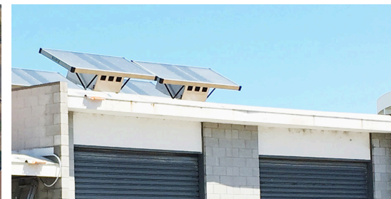
Project Solar PV, LED Lighting, Zero Mass Water Unit Client West Australian Police Scope Deliver energy efficient solutions Value $700K
