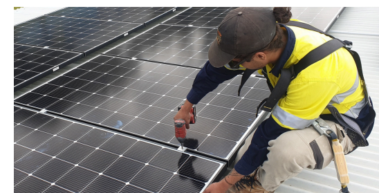
Project Sustainable energy for social housing Client Synergy Scope Install solar PV as a trial on 500 State Housing Properties Value Ongoing
