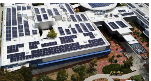
Project 310kW solar panel installation Client Water Corporation Scope Installation of 688 solar panels (310kW) Value $1.3M
