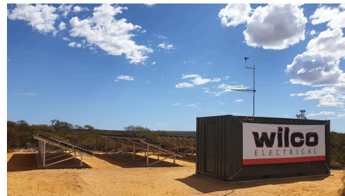
Project Kalbarri Skywalk National Park Client Dept Biodiversity, Construction & Attractions Scope Stand Alone Power Supply Value $160K
