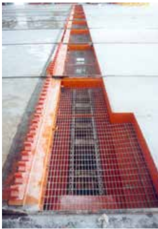
Debris conveyor chain
