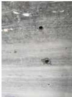
Detail of weep holes at the bottom surface of the concrete element
