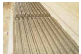
Exposed steel mesh
