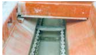
Debris conveyor chain
