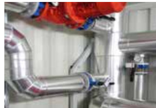
Insulated aluminium pipes
