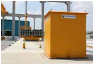
Concrete element transport line
