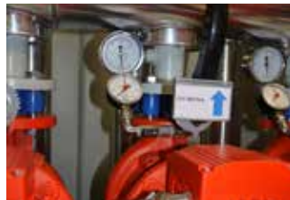
Pressure gauge with ball valve (in-flange type) for each production bed
