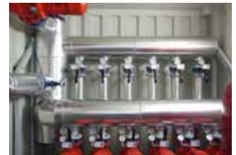
Primary pumping circuit manifold
