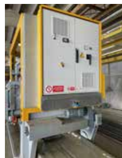
Electric cabinet protection
