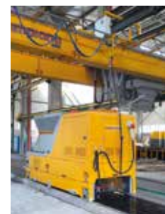
Electrical supply from the concrete distributor
