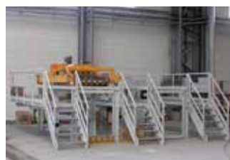
Service platform in the production area
