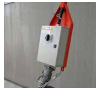
Electrical panel with power supply socket for the production machines
