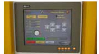
Large touch screen control panel
