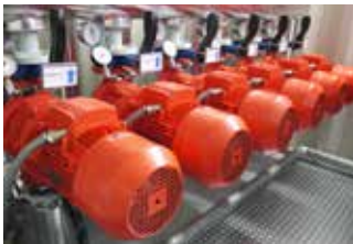
Pumps for the secondary pumping circuit to the production bed
