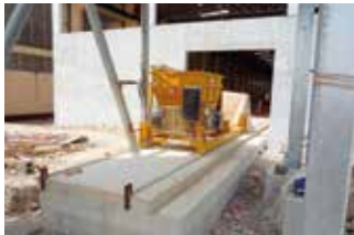
Trolley during the bucket transport from the batching plant to the production area
