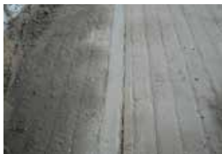
Worn concrete bed
