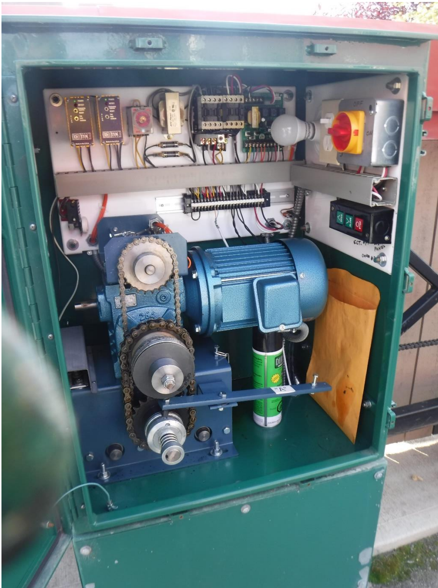
The front gate motor and control mechanisms.
