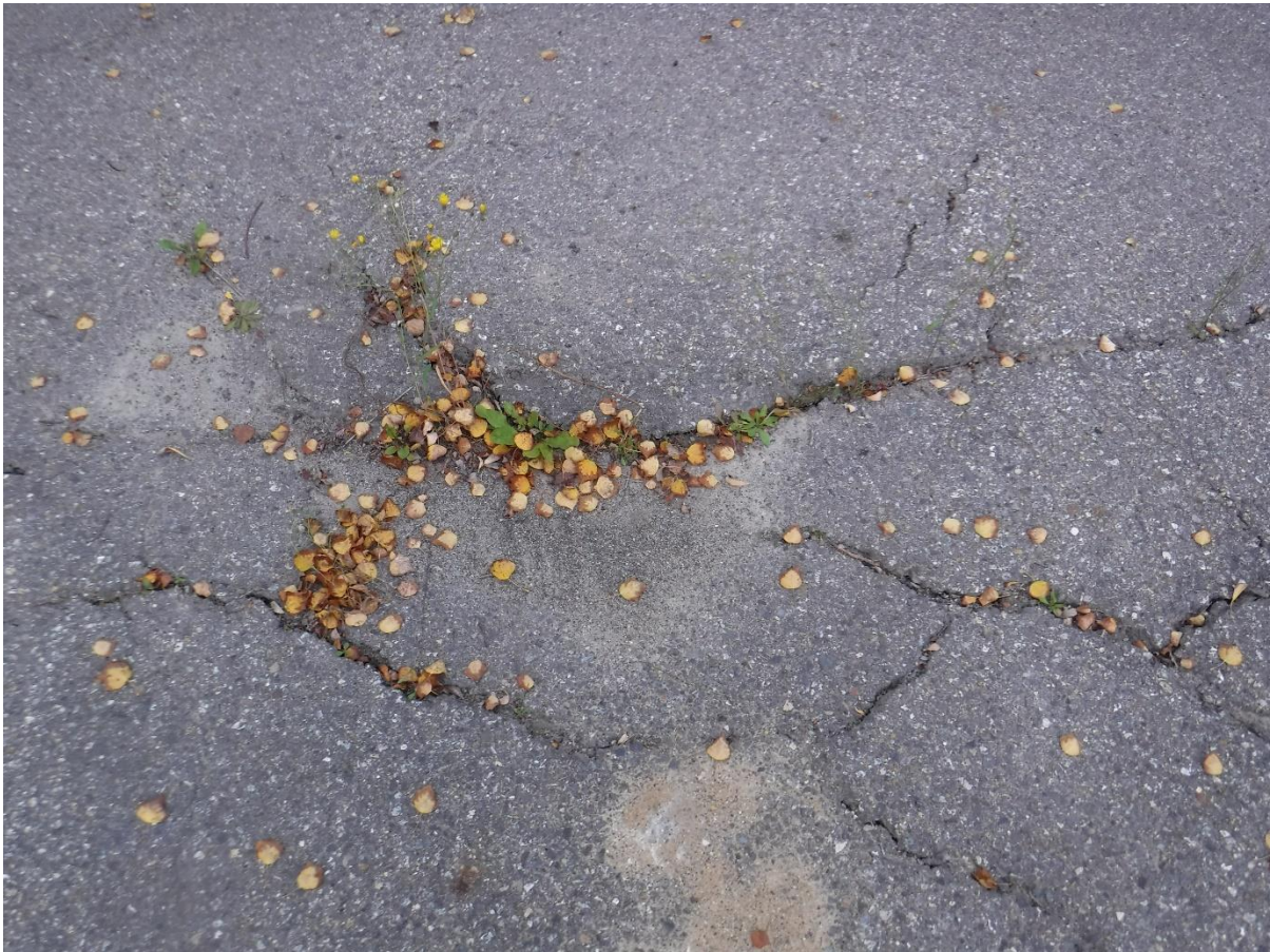
An area of subsidence in the asphalt. Now cracks have appeared and weeds are starting to grow through the cracks.
