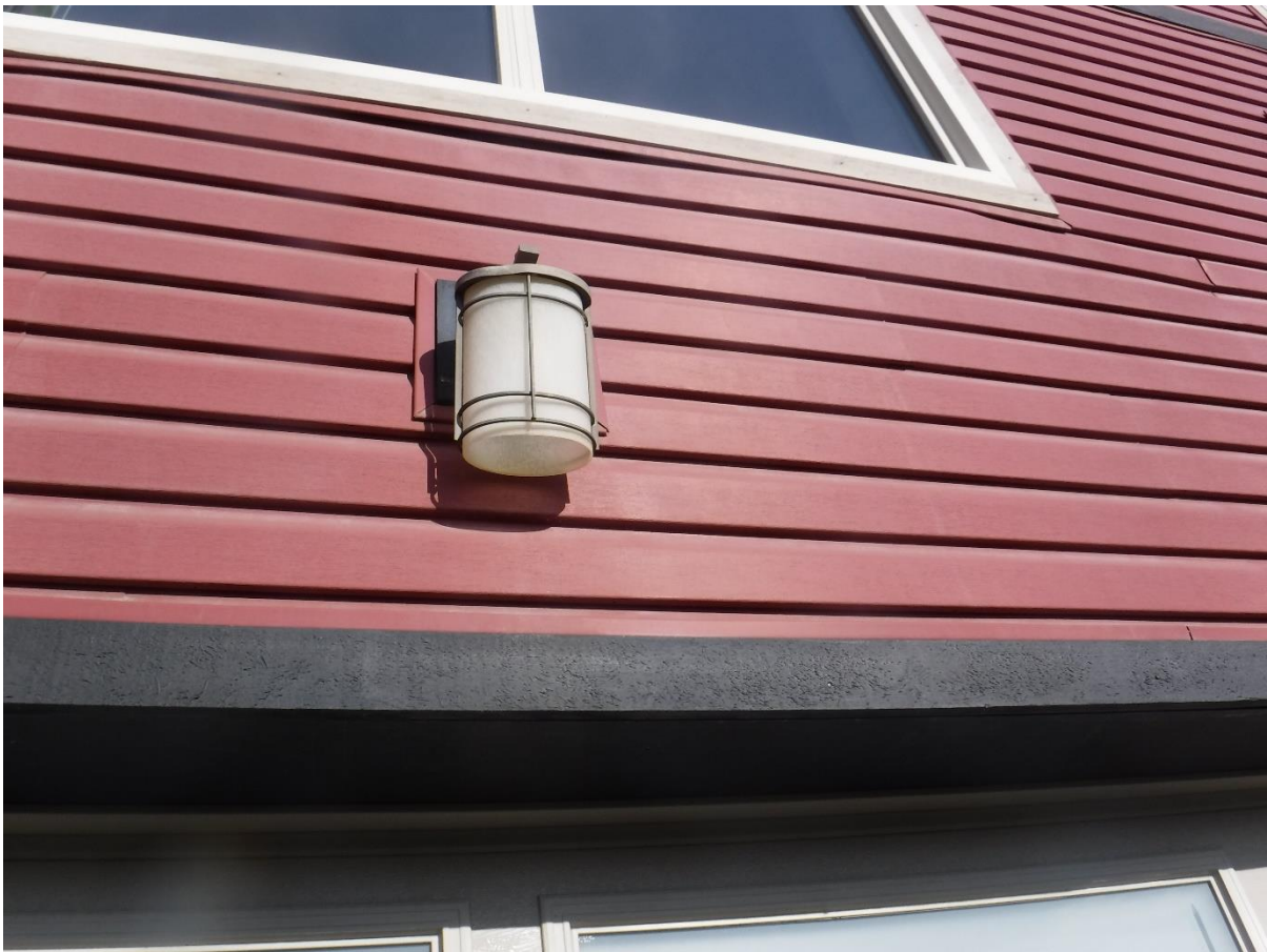
An outdoor light at the side of a building.
