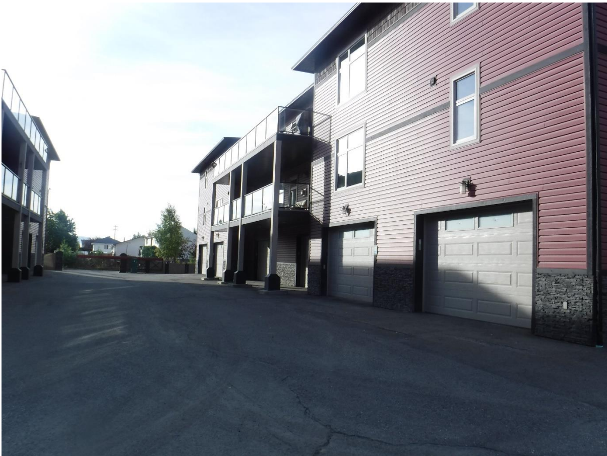
Same shot, but with Building B visible on the right. Cracks visible.
