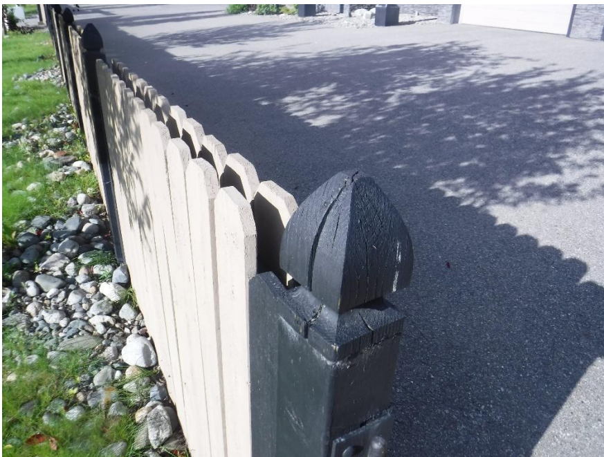
Big cracks in this fence post top.
