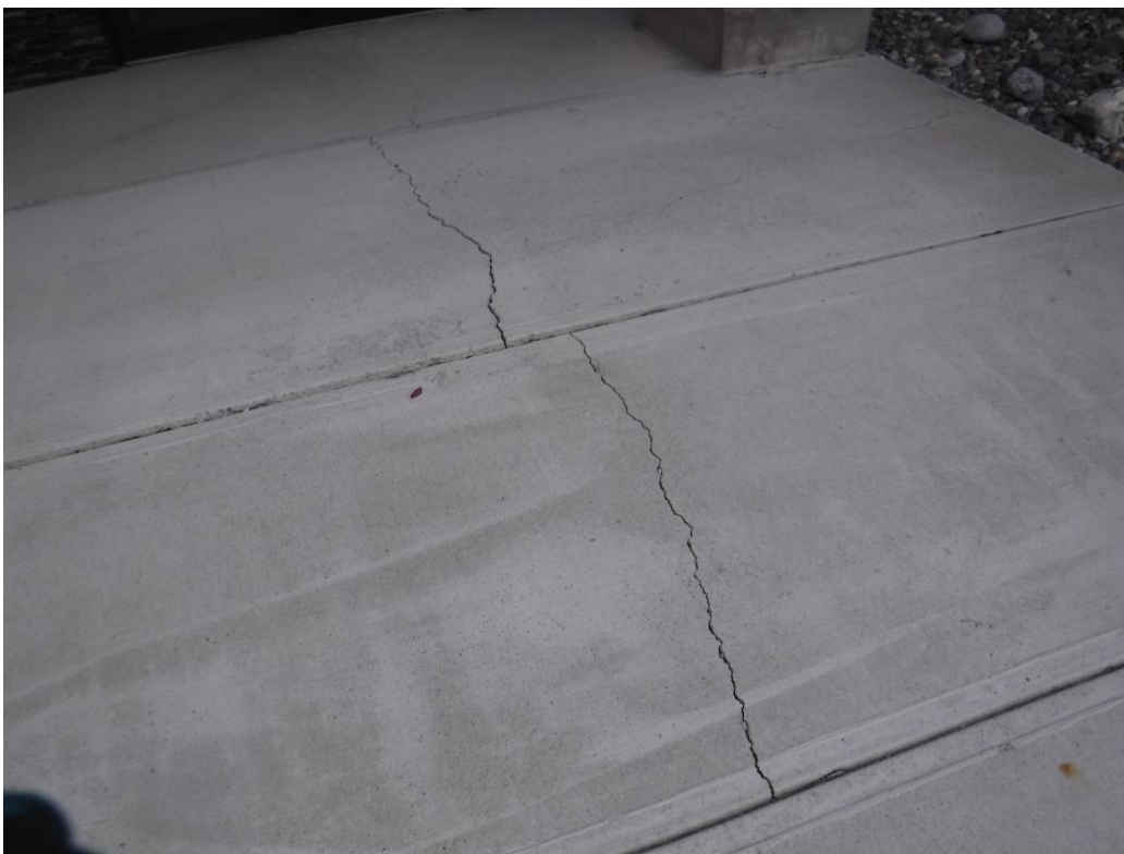
Small cracks in the sidewalk by a front door.
