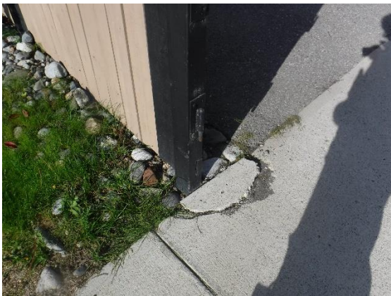
Damaged sidewalk by a gate post.
