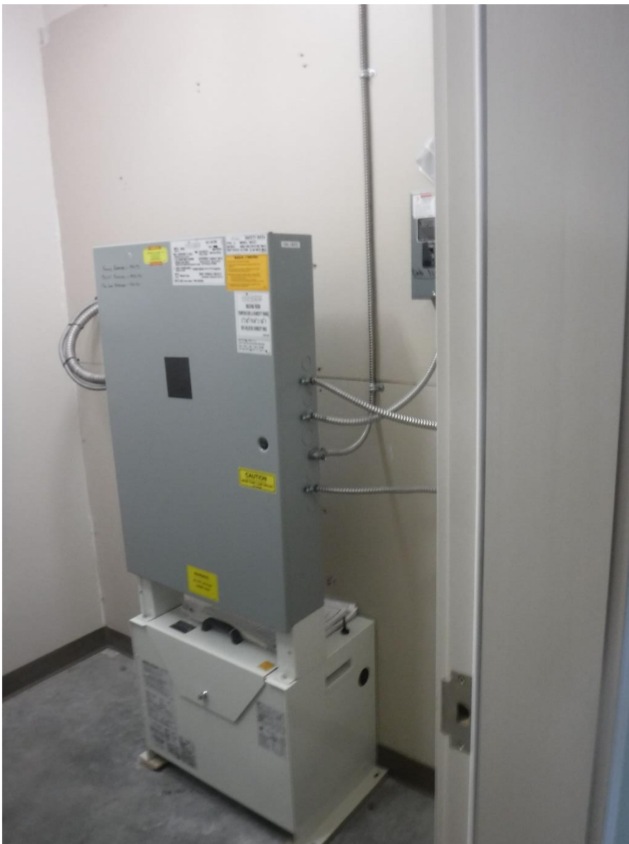
Electrical components associated with the elevator.
