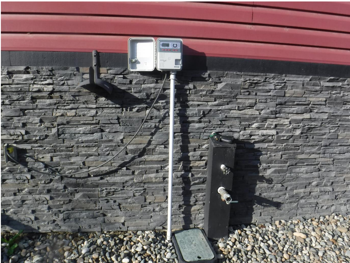
The control panel for the watering system.
