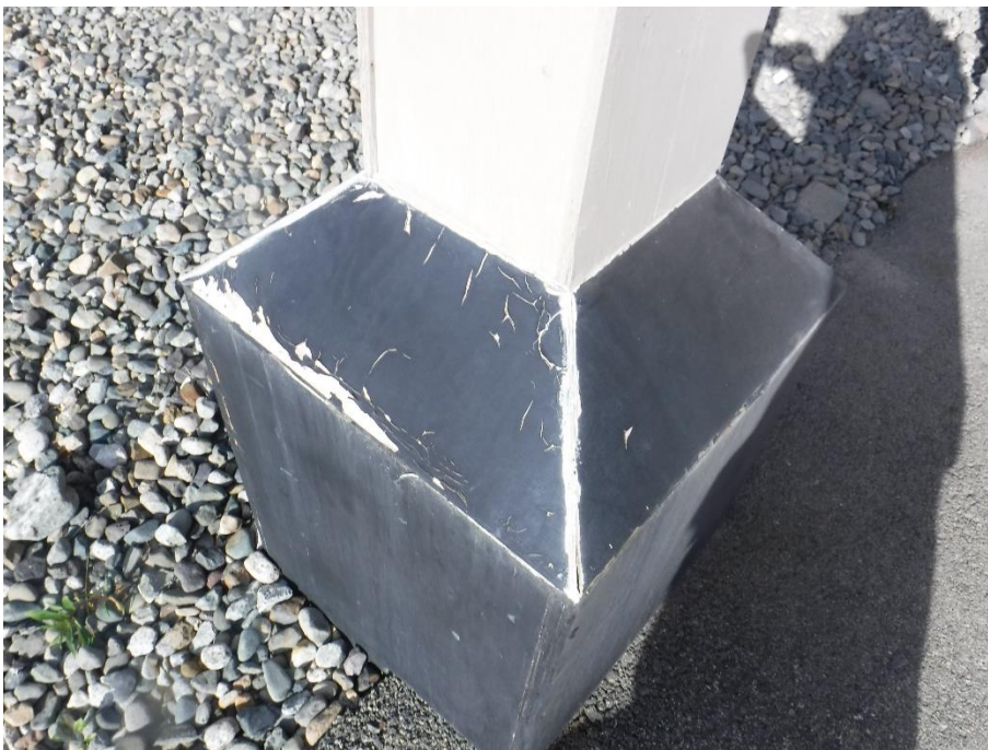
A south-facing post. The paint is peeling away. The south facing trim surfaces wear more quickly.
