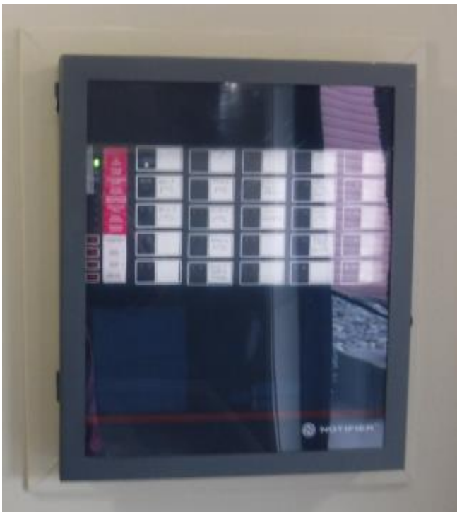
Fire panel at the front door.
