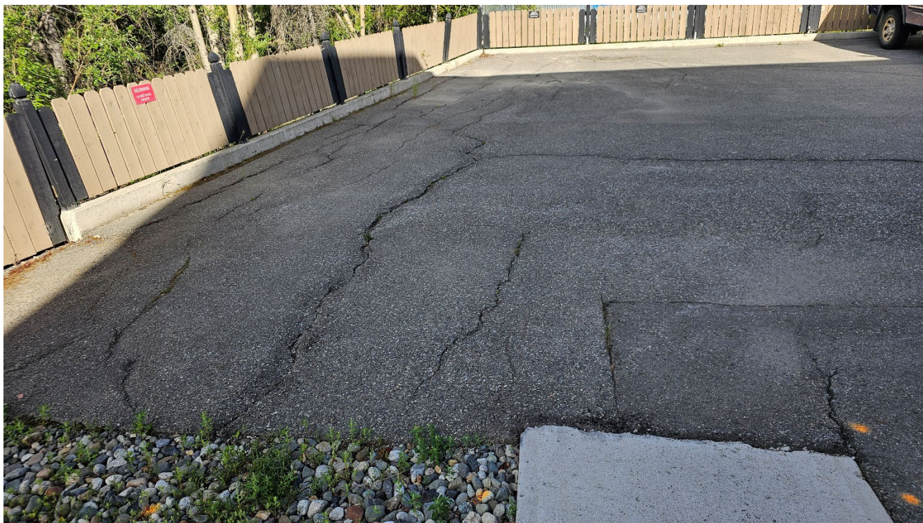
Photo 1: Pavement cracking in northwest corner
