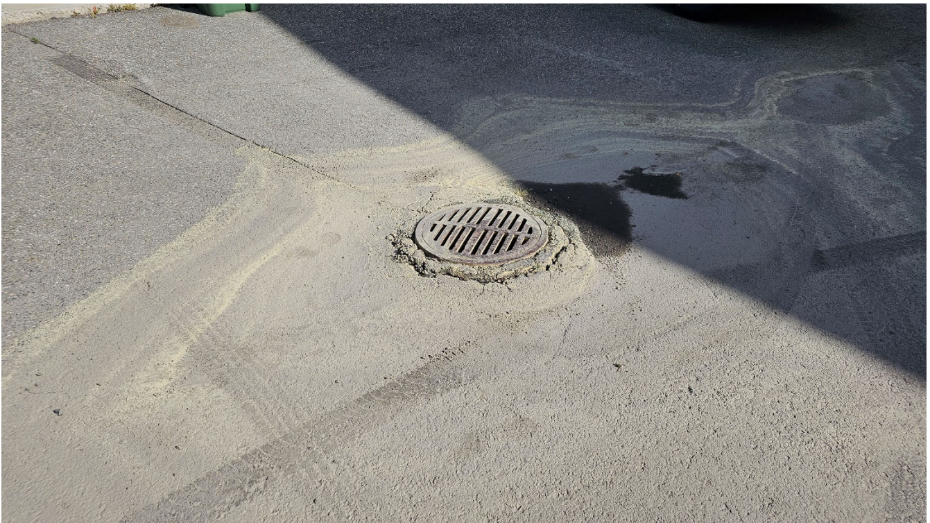
Photo 3: Heave/settlement around northern catch basin
