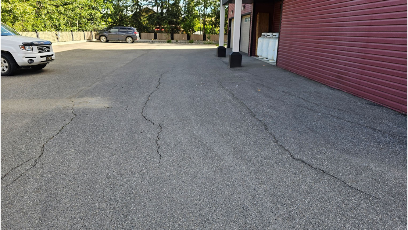
Photo 4: Pavement cracking continuing towards borehole BH23-02 with BH23-03 in the foreground
