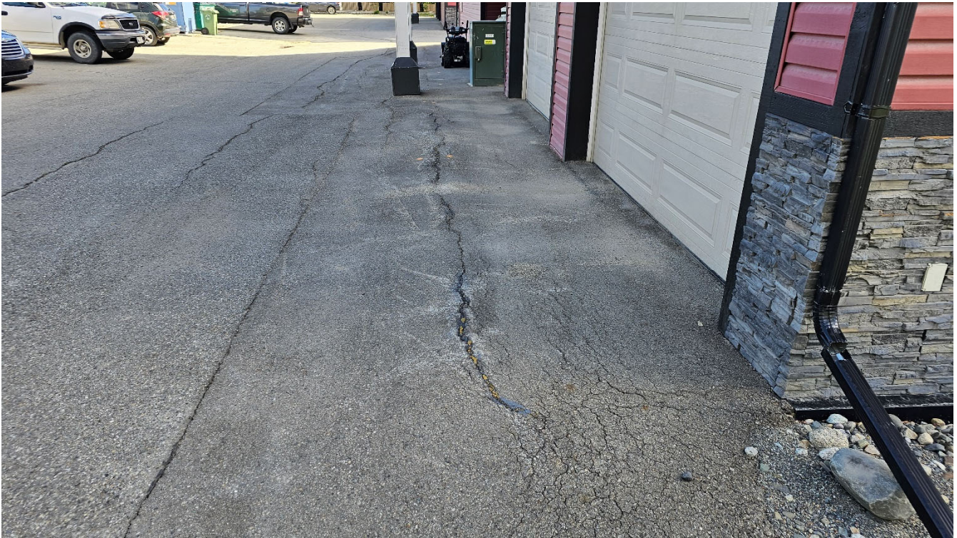
Photo 2: Pavement cracking along 2012 remedial repairs
