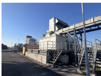
Generator set enclosure and inlet filter house
