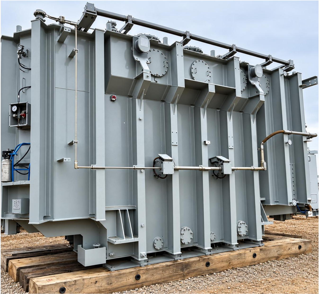
Main tank as stored — oil-filled under nitrogen blanket; accessories stored separately.
