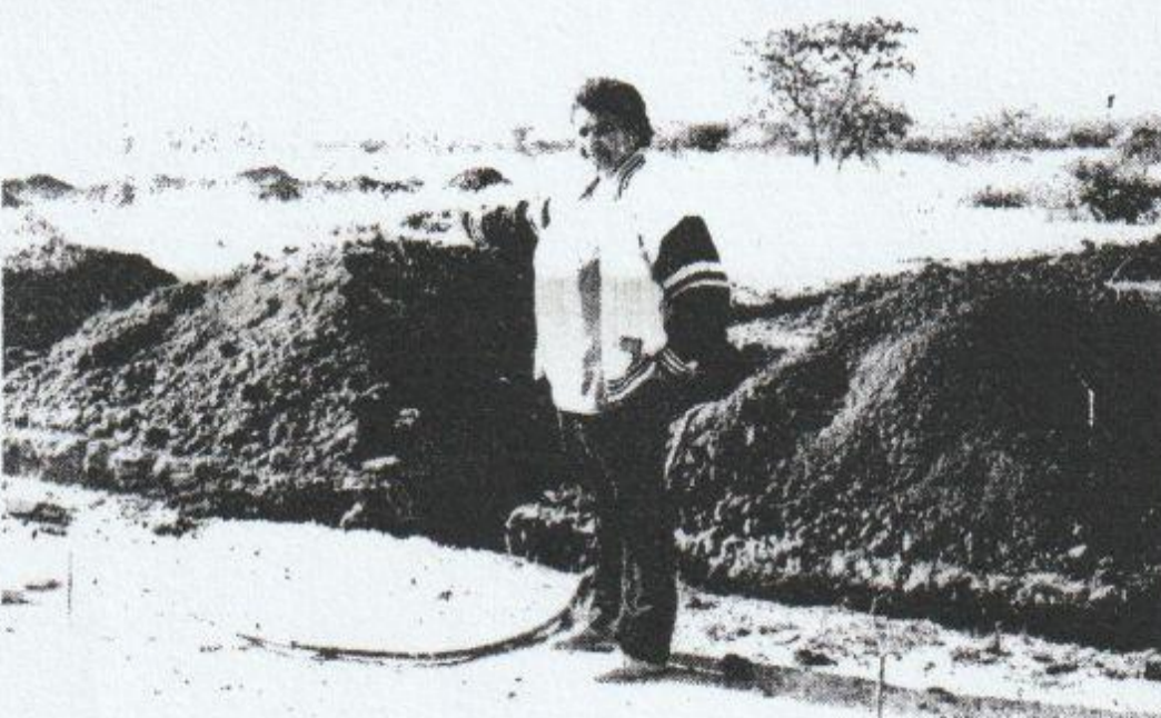
Betty Kennedy is the brain behind Betty's Day and Night Care Centre which also resulted in the establishment of another private school for Pietersburg. Here she is pictured at the foundations for a storeroom, coldroom, laundry and kitchen.
