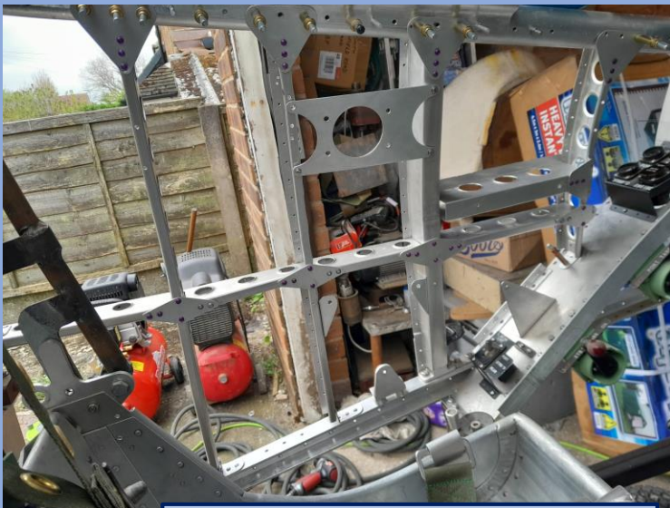
All the port frames to intercostals, lower longeron and upper longeron fish plates now fully riveted up. Sub frame for the throttle box fully fitted. Starboard done, too.
