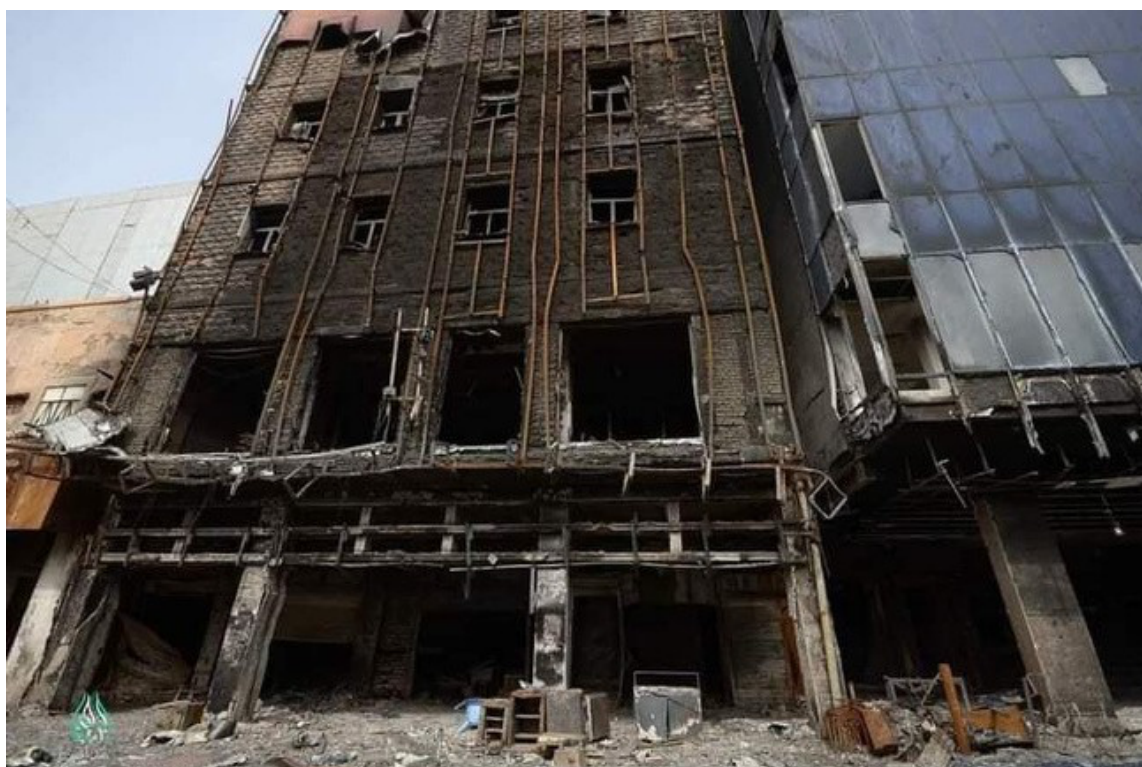
Destroyed government facility by the 15 April 2023 war
