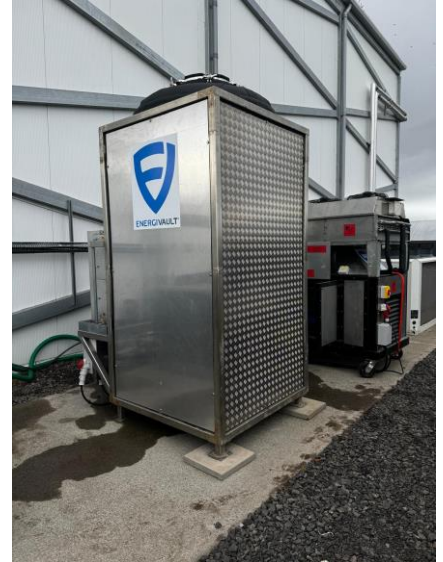
Propane charger and store demonstration unit, installed at IGS.
