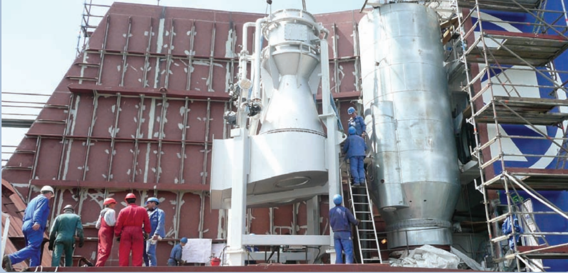
Figure 11: The 21MW hybrid scrubber during installation on Ficaria Seaways (image courtesy of Alfa Laval)
