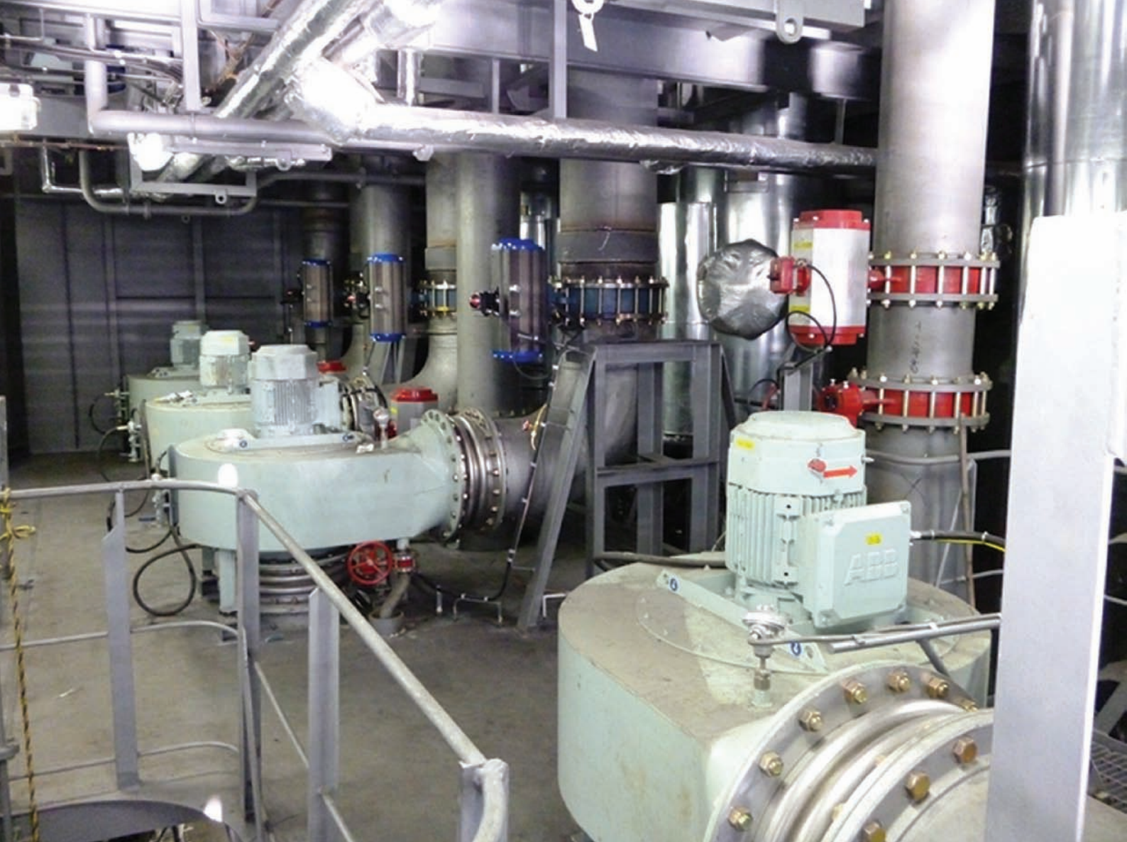
Figure 6: ID fans in exhaust ducts (image courtesy of Hamworthy-Krystallon)
