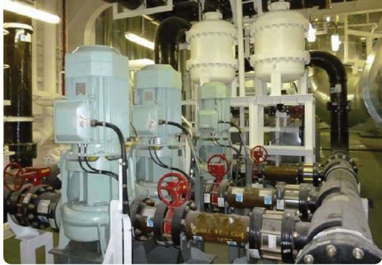
Figure 12: Washwater treatment system with GRE piping (image courtesy of Hamworthy-Krystallon)
