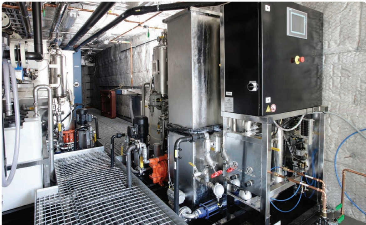
Figure 13: Multi-stage washwater treatment system used with closed loop SO x scrubbers (image courtesy of Wärtsilä)
