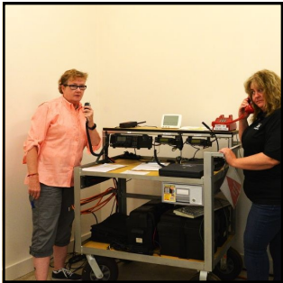
Beth Mason, KE7CRL Facilities Technology Specialist, and Jackie LaVerne, Emergency Coordinator, both of Evergreen State College in Olympia are testing the radio equipment at the Emergency Communications Center.
