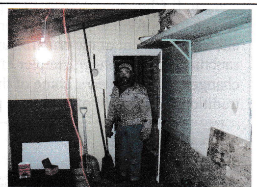
Kevin Ferden begins process of installing electrical wiring, sockets, switches for the work area.
