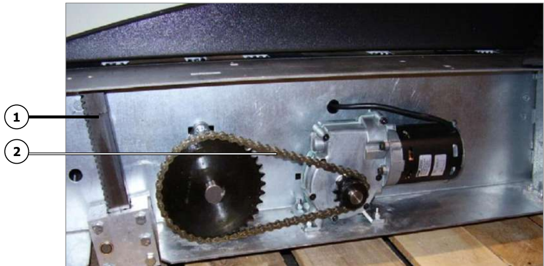
Fig. 117 Lubrication, incline system
