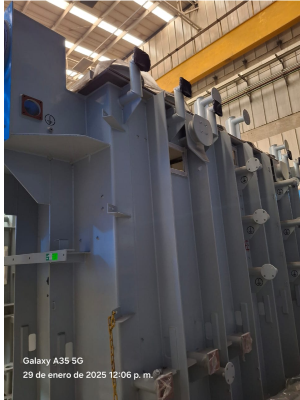
Photo 1: Transformer tank — radiator bank side view, showing radiators, grounding connections, and protective covers
