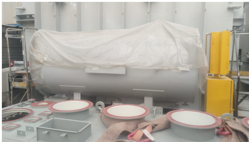
Photo 4: Top of transformer showing conservator tank (covered), bushing openings with protective covers, and lifting provisions (Jan 31, 2025)
