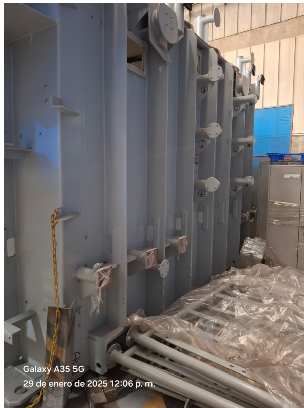
Photo 2: Tank side view showing radiator banks, drain valves, and packaged accessories (Jan 29, 2025)
