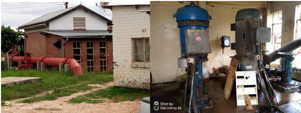
Figure 3.8.1.3.2: Hunyani Raw Water Pumpstation and Raw water pumps
